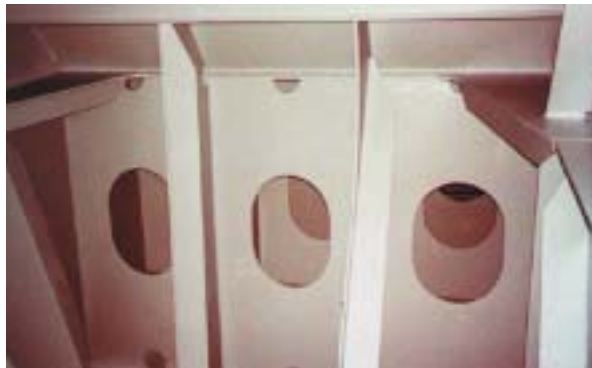
Fig. 1: Good edge retention is critical in ballast tanks.
